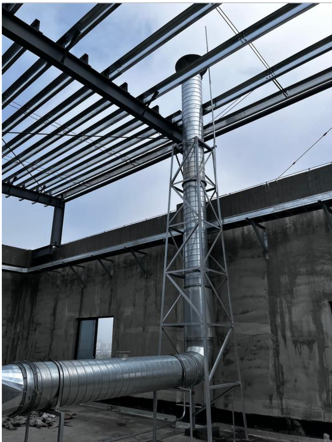
磨床粉尘排气筒
